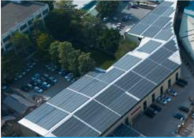
500kW On-grid and Energy Storage Solar Project on Our Factory
