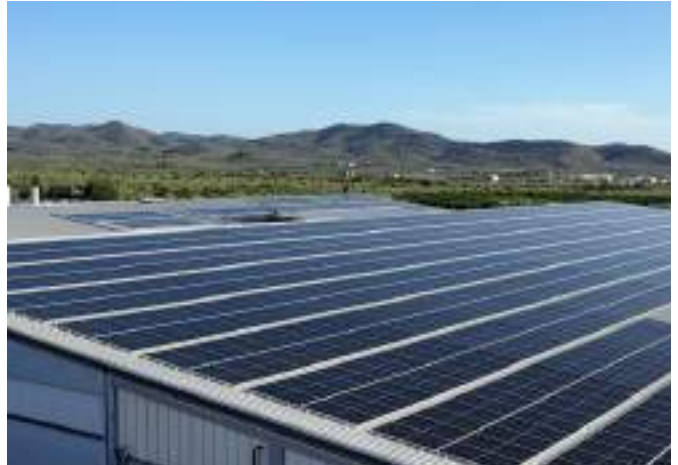
5MW On-Grid Solar Project in Shaoguan
