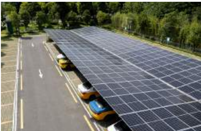
200kW Parking Shed Energy Storage Station in Guangzhou
