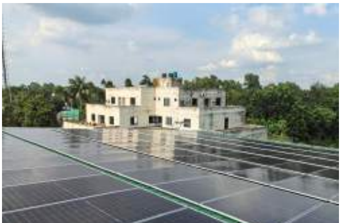
800kW Storage Project in Paluga, Bangladesh
